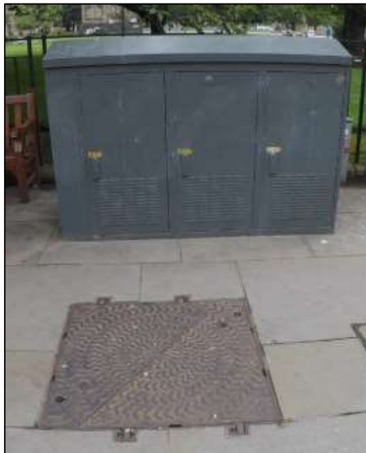
Figure 19: TEC cabinet (existing design)
