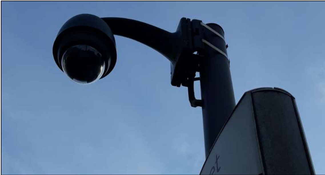
Figure 14: CCTV camera (existing design)
